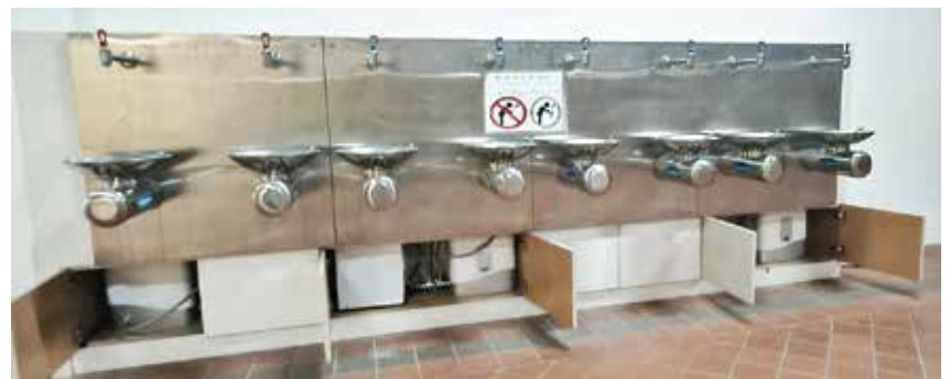
*Drinking water for government offices and schools
